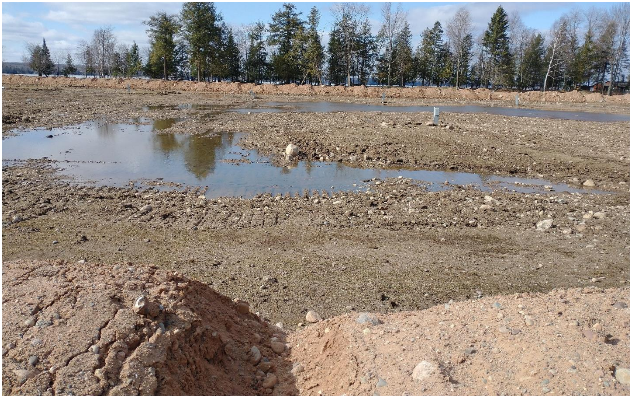
Photo 6 – Topsoil scraped east central campsites and road (under fill material) from southeast of Project Area facing north
