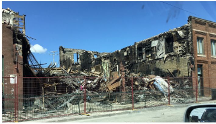
Damage in the "Uptown" business district of Kenosha
