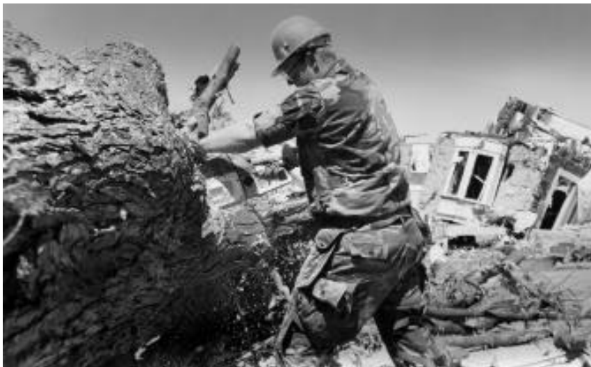
Company A, 724th Engineer Battalion, Wisconsin Army National Guard on Main Street in Oakfield, after a tornado destroyed much of the village of 1,000. (Larry Sommers, Wisconsin Department of Military Affairs)
