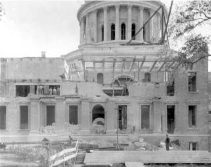
Workers demolished the north wing of the old capitol in 1913 to make way for the final phase of the current structure; the dome of the new building (background) was already complete. (State Historical Society, #WHi (X#) 52940)
