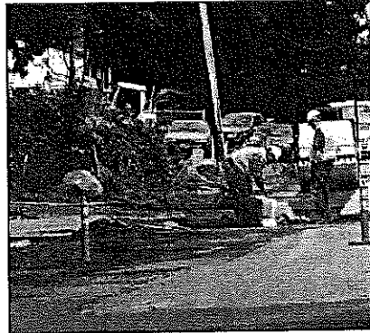
As pavement conditions deteriorate, maintenance and repair costs become increasingly more time intensive and costly.
