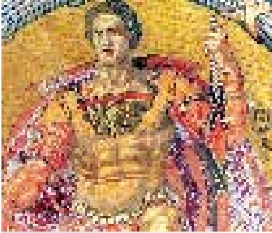
Portions of Kenyon Cox's mosaics were repaired with an inferior adhesive, marring their appearance. (Kathleen Sitter, LRB)
