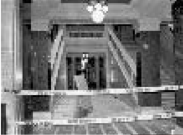
Areas of the capitol under renovation were closed to the public (left). Temporary plywood walls were erected to protect exposed surfaces (below). (Kathleen Sitter, LRB)
