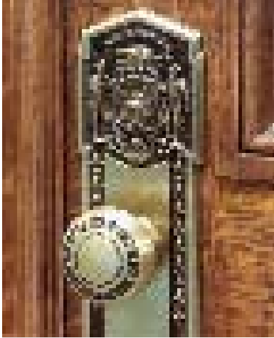
The effort to replace modern door-knobs with replicas of the original design in 1982 stirred controversy, but demonstrated a commitment to the vision of the capitol's architects. (Kathleen Sitter, LRB)
