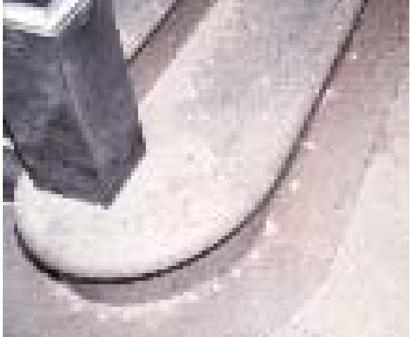
Damage caused by driving carpet nails directly into a marble floor. (Kathleen Sitter, LRB)
